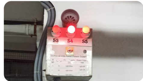
Pump room fire panel alarm system
